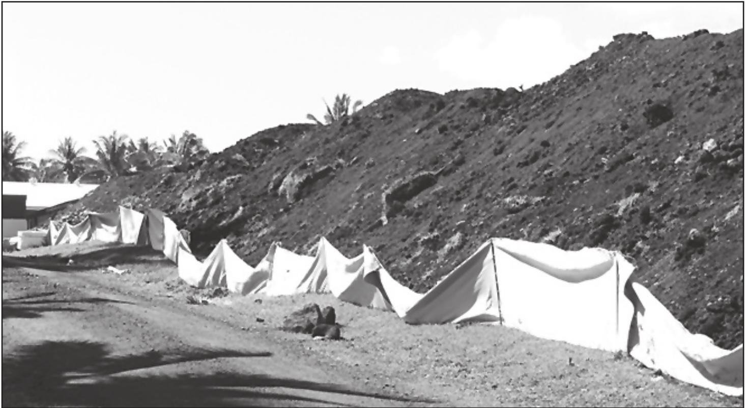
Use of silt fences on the construction of the multi-complex by T&M contractors
